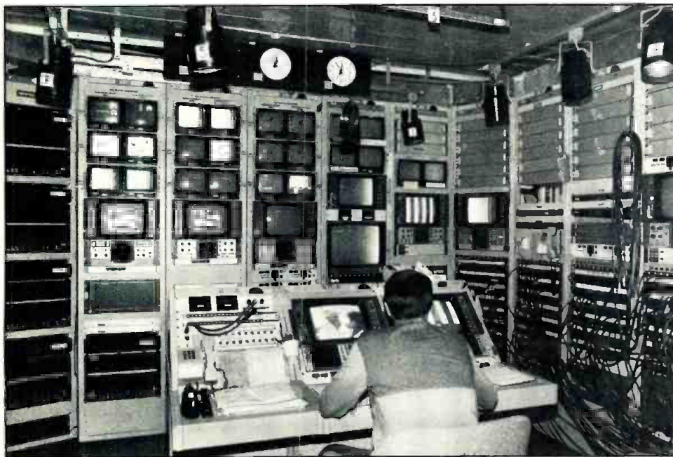
ABC's Olympic control room
